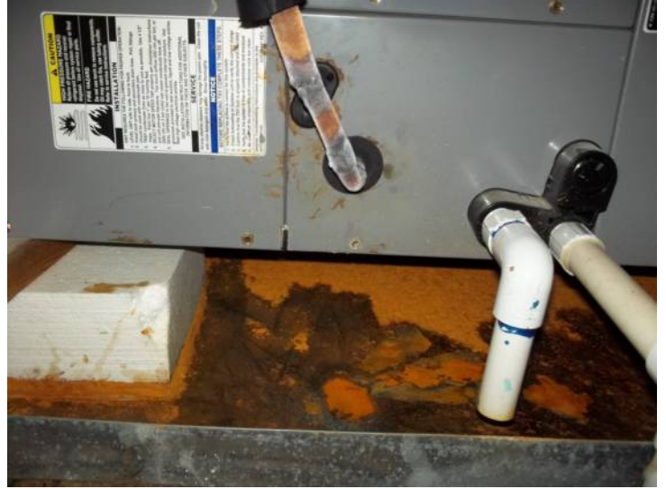
Rust stains are visible in guest air handler pan, refrigerant line insulation is short at unit casing.
