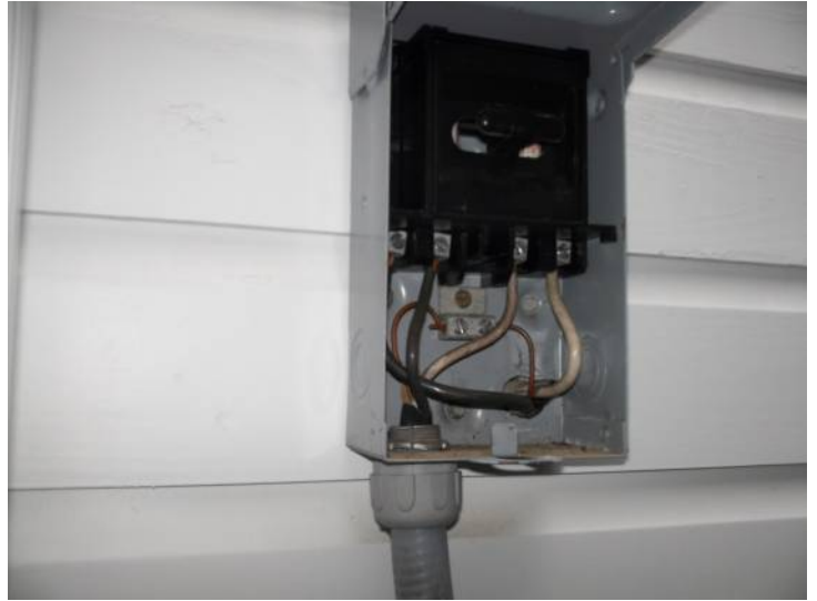
Furnace disconnect inner cover is missing at right side of structure.
