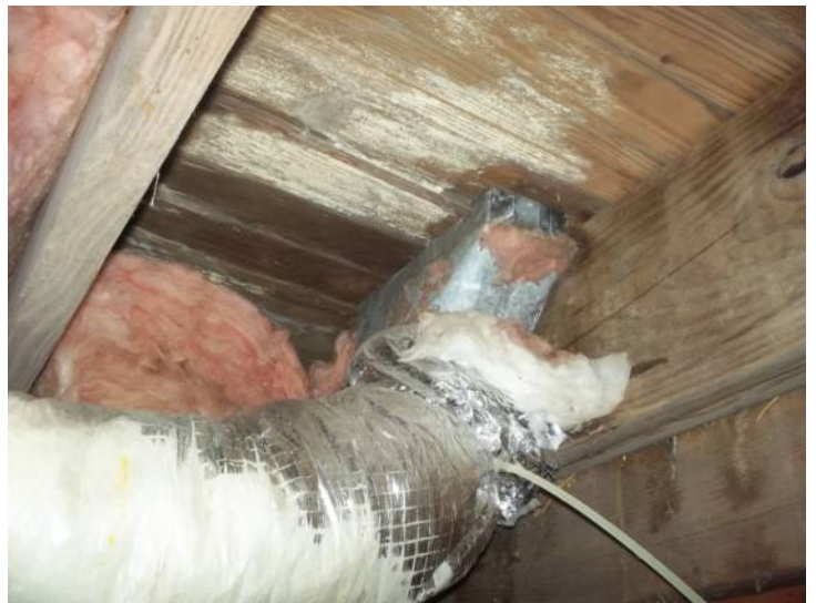
Stains and deteriorated sub flooring are present around floor registers where duct connection is partially detached.
