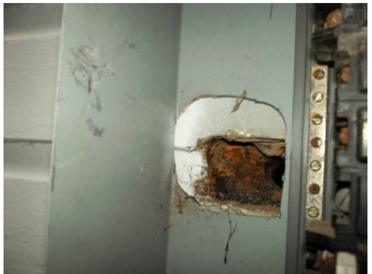
Holes present at rear of exterior service panel needs to be covered.
