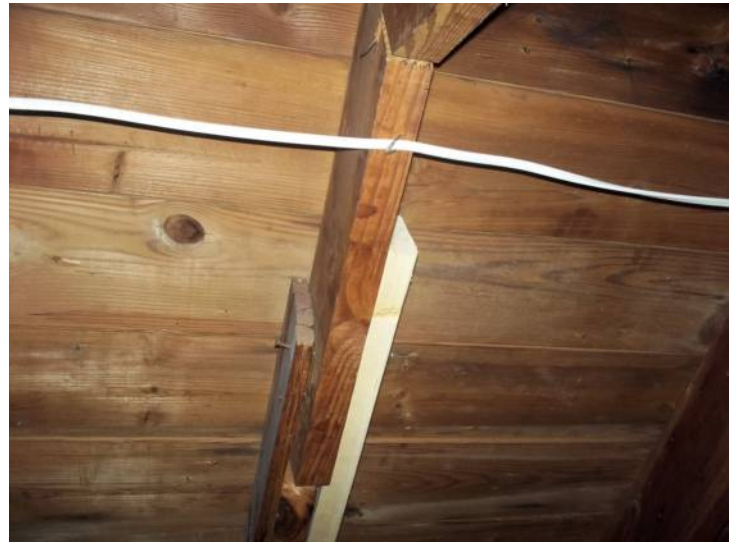
Rafter splices present above middle hall and at right front are not properly reinforced.
