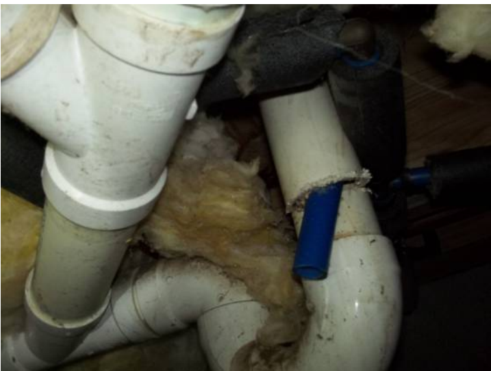
Drain pipe under master shower has been severed.
