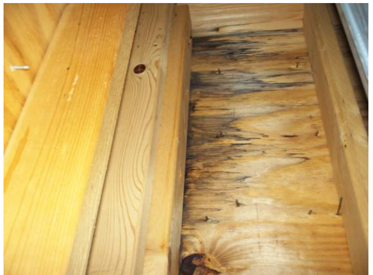
Living room chimney stucco exterior has stains present in chase at top by cover.
