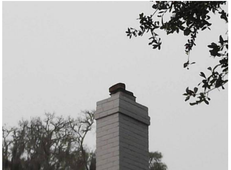
Right chimney flue cover is held in place by a brick, flue is blocked and currently unsafe to use.
