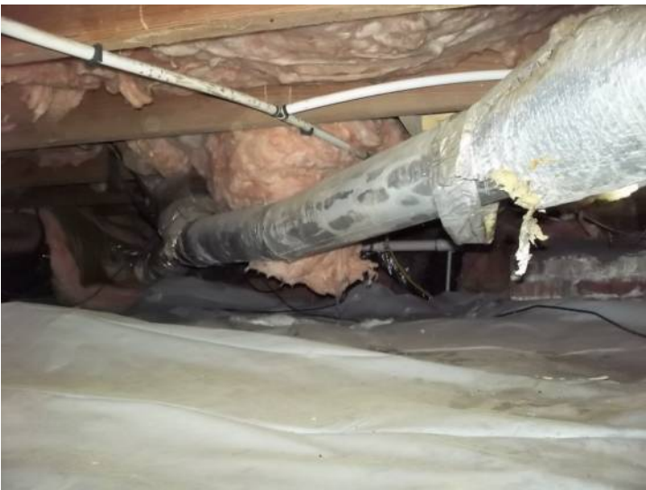
Crawl space ductwork insulation is absent under rear hall at original structure.
