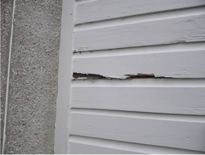
Rotted wood observed at siding at front of left rear chimney, caulk filled backer rod expansion joint absent chimney and siding.
