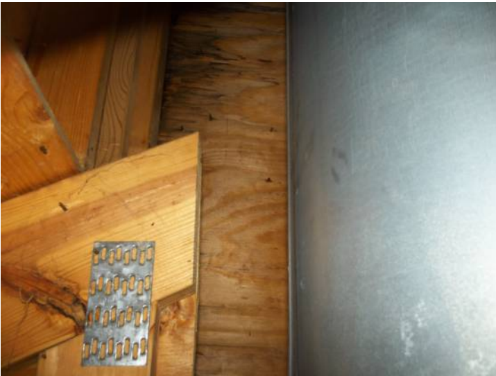
Truss member has been cut to accommodate living room fireplace flue, stains present in chimney chase at wall sheathing.
