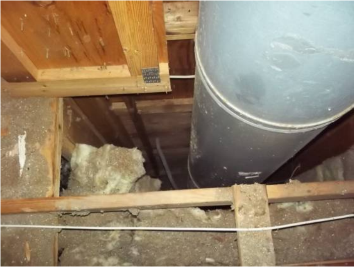
Chimney chase is open to the attic, truss has been cut.
