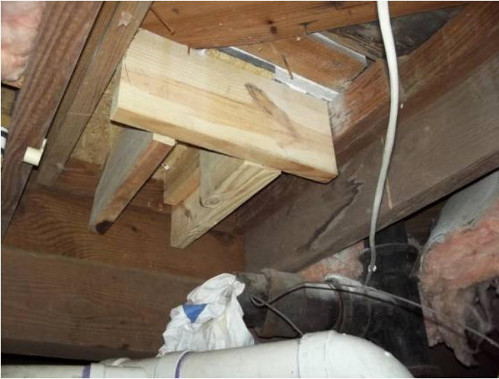
Ends of joists under front left bedroom bath, and the short header that supports them, do not have bearing on hangers or ledgers.
