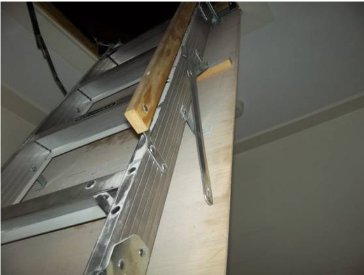
Pull down stair front hinge arm is detached.
