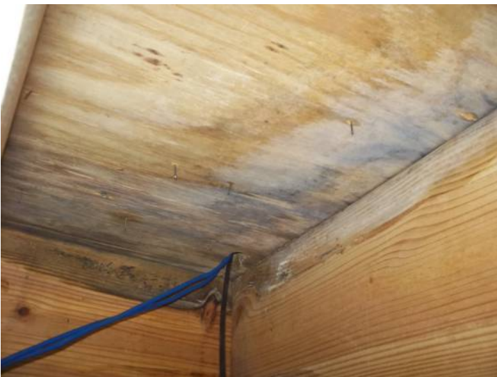
Water stains are present on sub-floor in rear crawlspace at left front corner of living room by side entry door.
