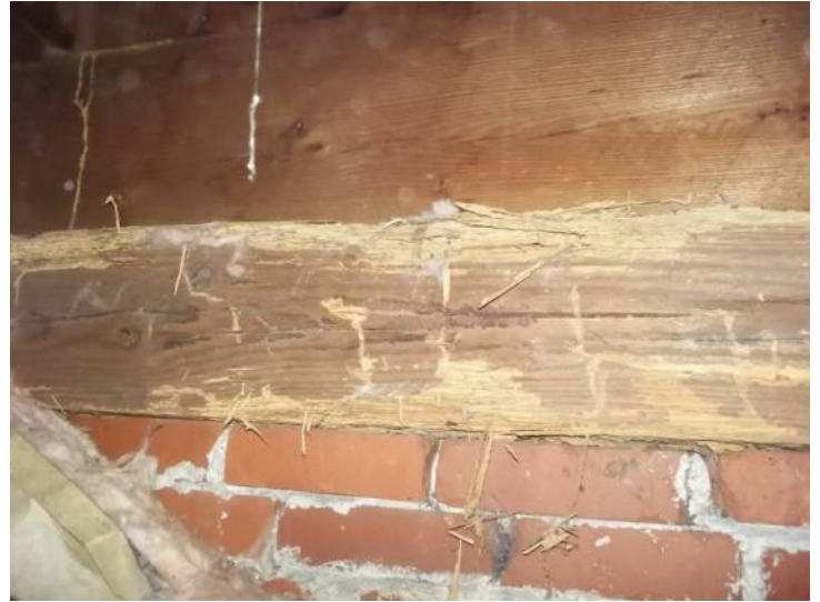
Banding along left side of original structure are insect and moisture damaged.
