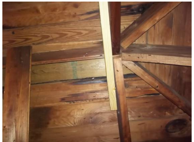
Stains present at middle hip ridge. Hip ridge is not supported.
