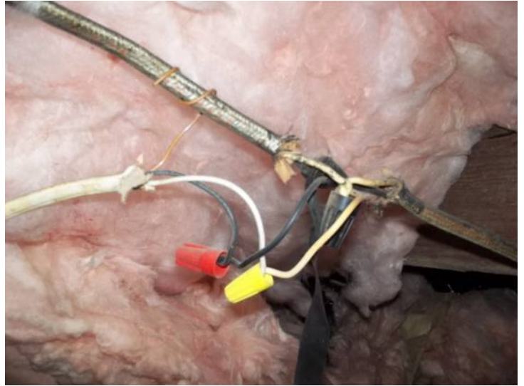
Exposed slices at cloth romex wiring in middle area of crawlspace below hall to right front bedroom.
